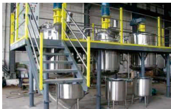
Silicone oil tank
